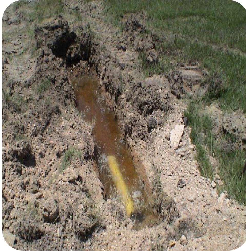
Ground water collected by a french drainage system
