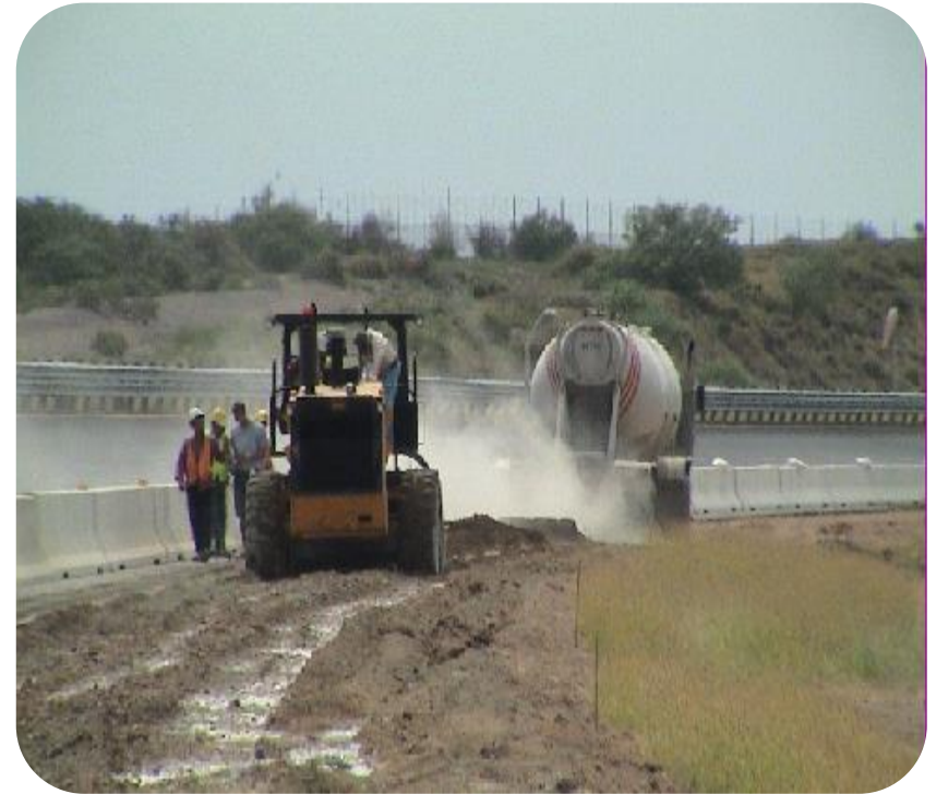
A silo truck is distributing the cement powder by the use of spray bar
